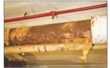
Corrosion under Insulation
