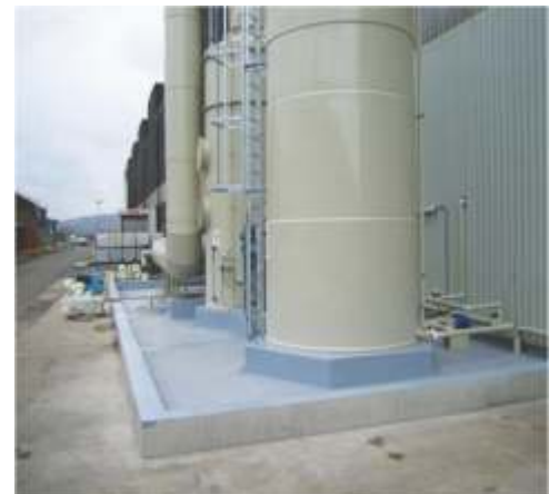
Acid storage area bund lining
