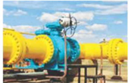
Metal Pipe & Flange Connections
