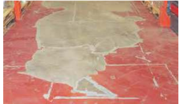
1311 MVT will not peel off due to osmotic pressure
