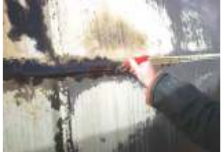
Application on rusty /damp surface
