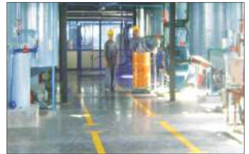
Lube Oil Plant
